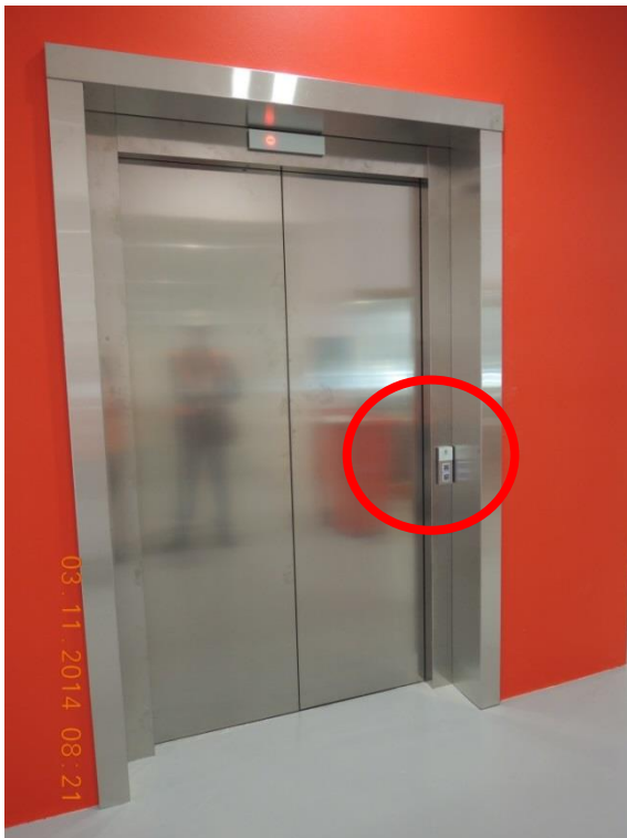
Figure 8 image of non-compliant lift call button installation
